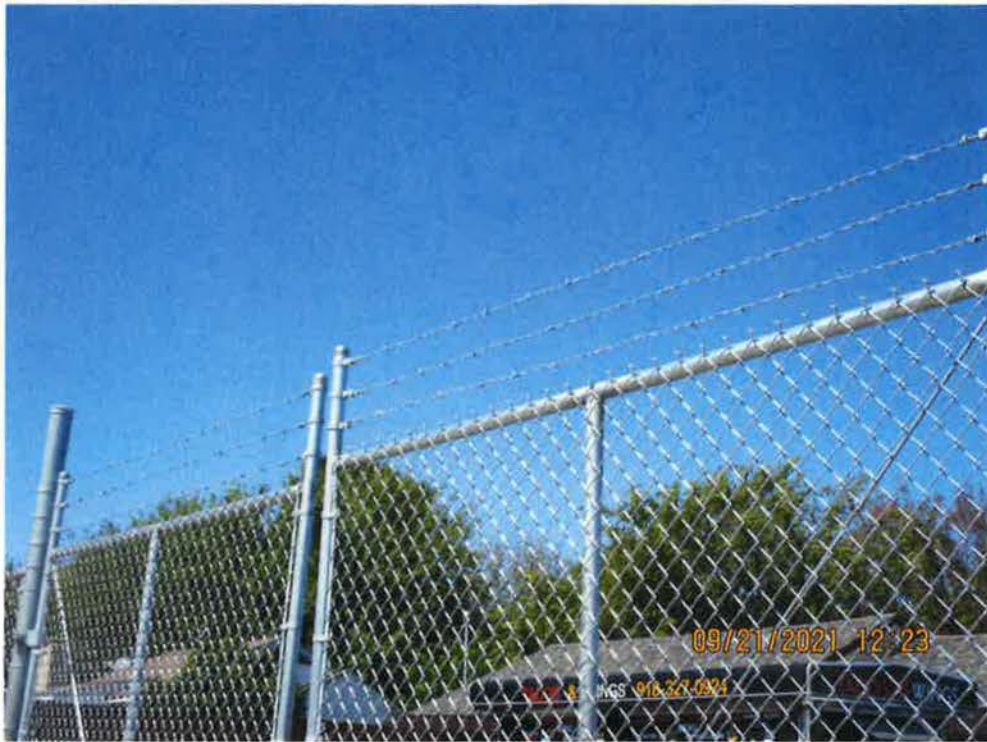
Barbed wire is still located on gate
