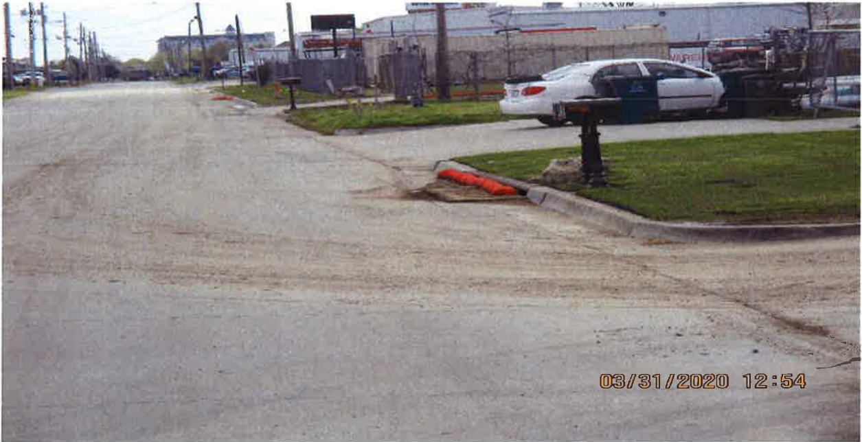
Gutter on 107 th E Ave.
