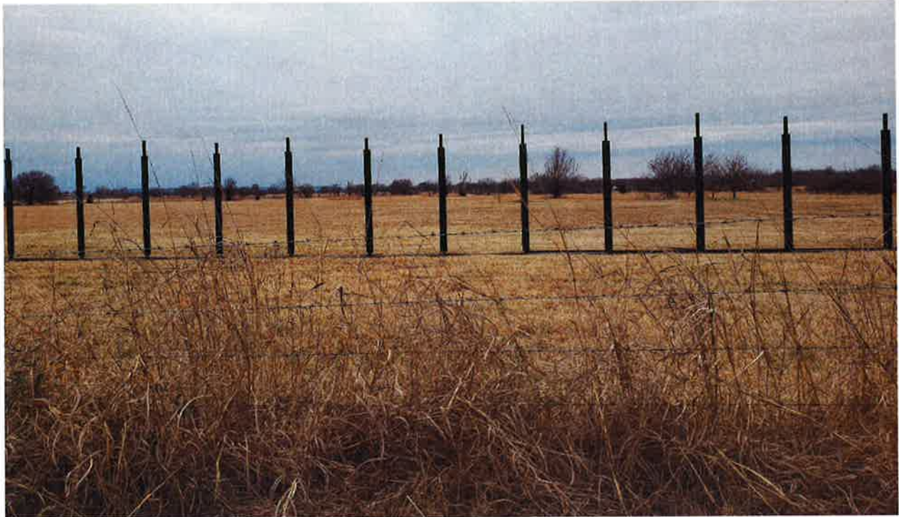
Looking west toward subject property from North Sheridan Road where the fence installation began in the front yard
