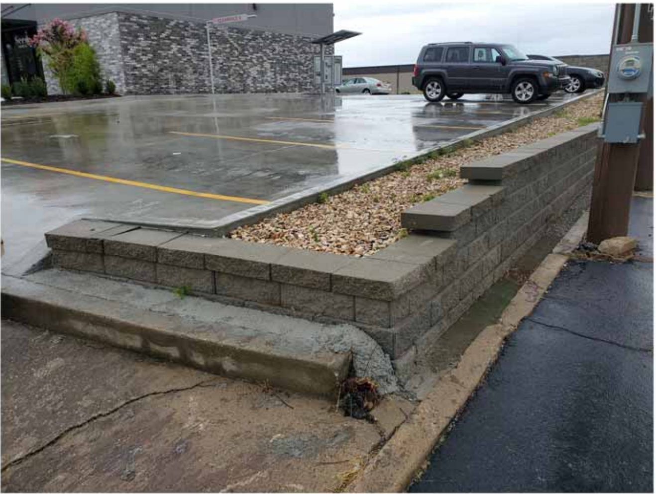
The lowest part of the retaining wall. Still too high to climb. West end of the wall, looking east north east
