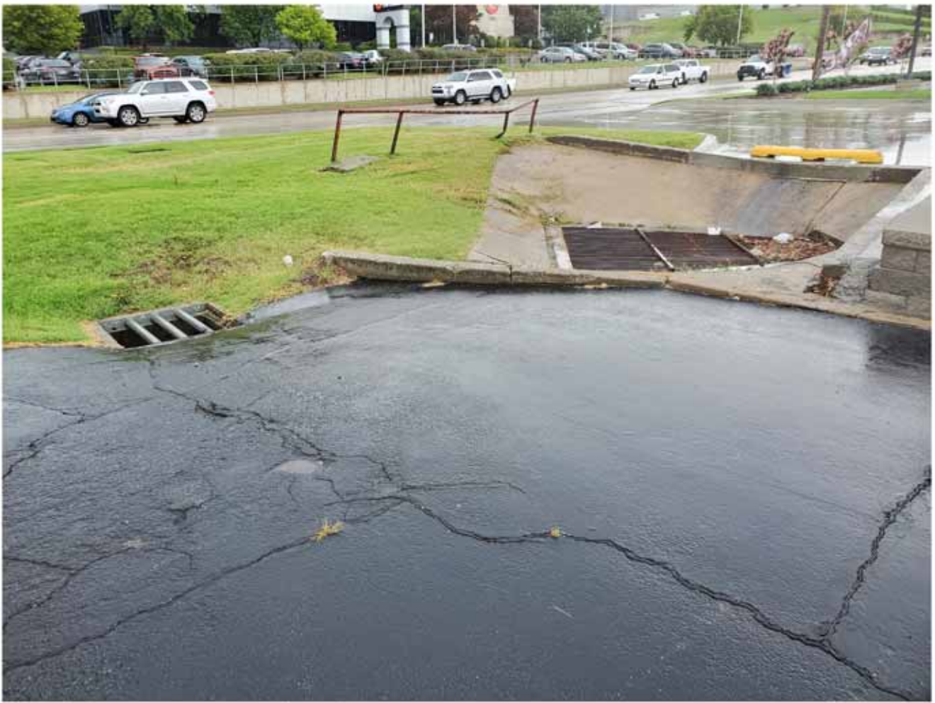
A drainage culvert & drains at the N.W corner of the parking lot at Last Call
