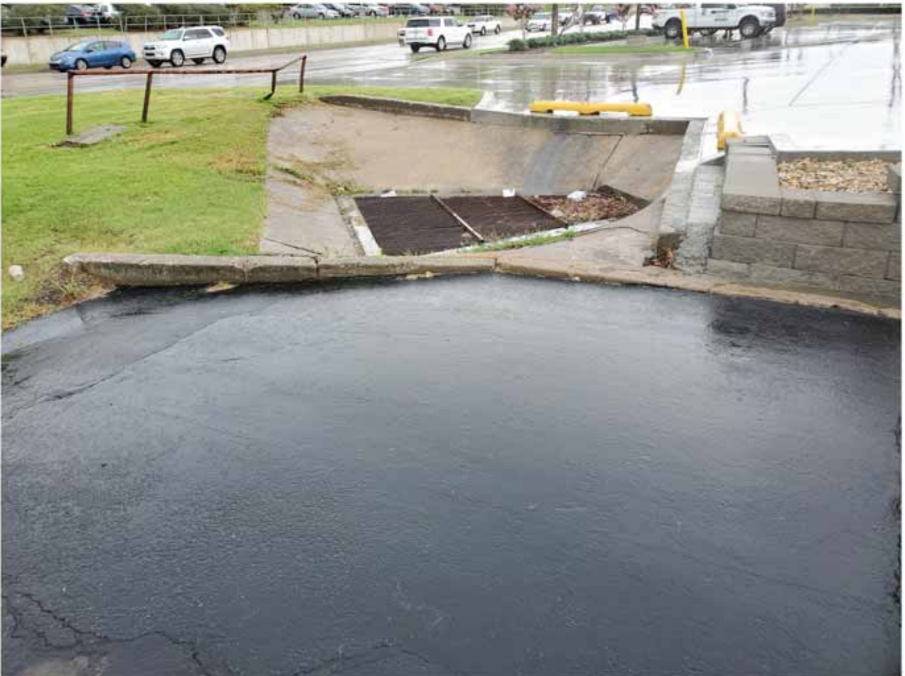
A drainage culvert & drain at the N.W corner of the parking lot at Last Call
