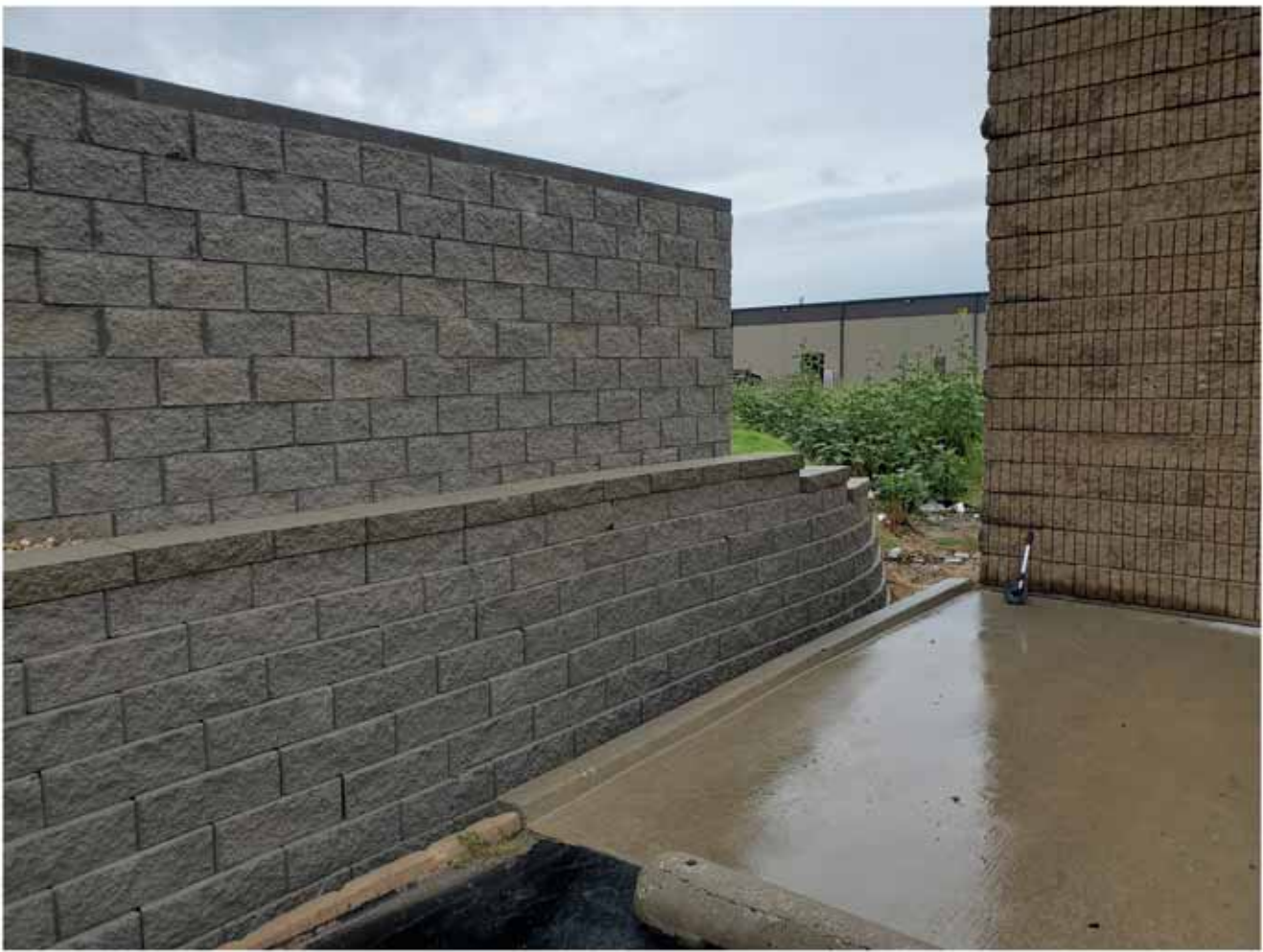
East end of the wall and the corner of Last Call, looking NE
