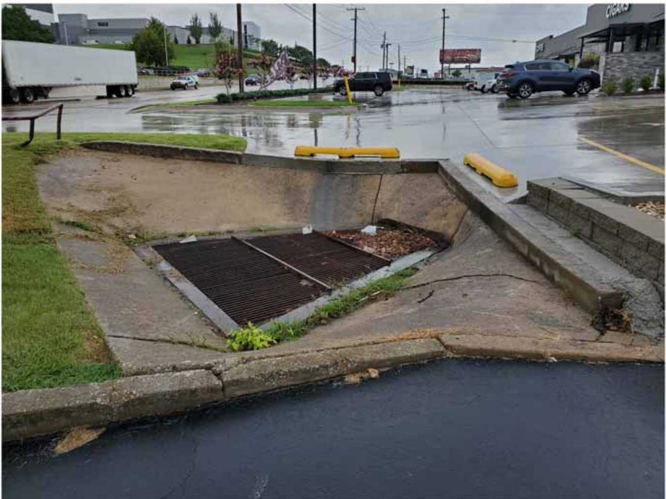
Drainage culvert & drain at W end of the retaining wall, looking north.
